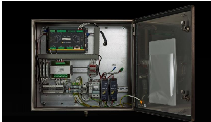
Figure 2 - Smart device in substation. It both talks to intelligent unit and control center over radio network. Intelligent unit measures current, voltage, power and other important parameter and sends them to smart device. It also detects faults on guidelines and use protection function to protect substation. All information from smart device are sent to control center.
