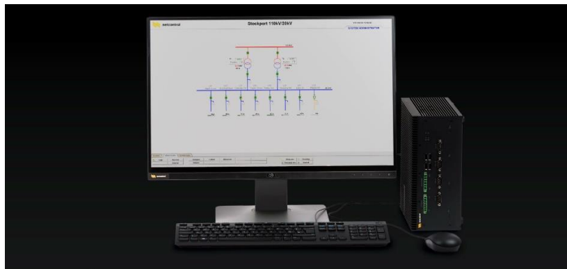
Figure 1- SCADA system in control center. It represents different analog and digital parameters collected from automated substations. It also enables human operator to remotely control substations.
