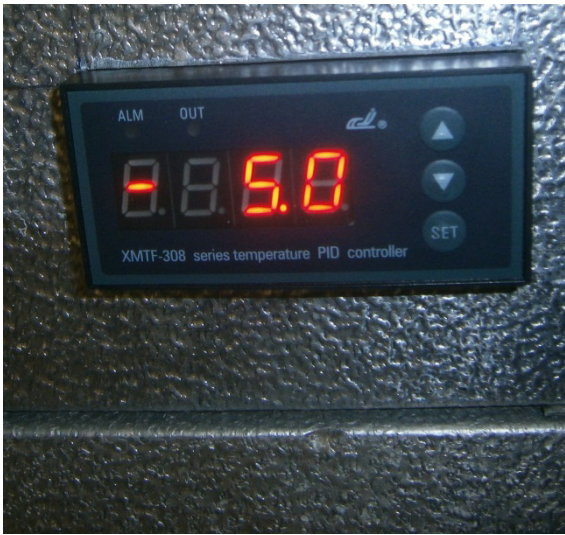
Fig. 3. The sensor for maintaining the temperature inside the test chamber
