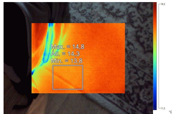
Figure 27. Floor above unoccupied flat
