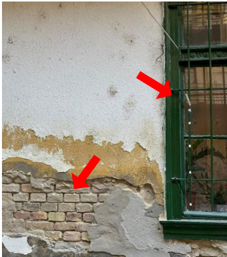
Figure 6. Sensors placed outside
