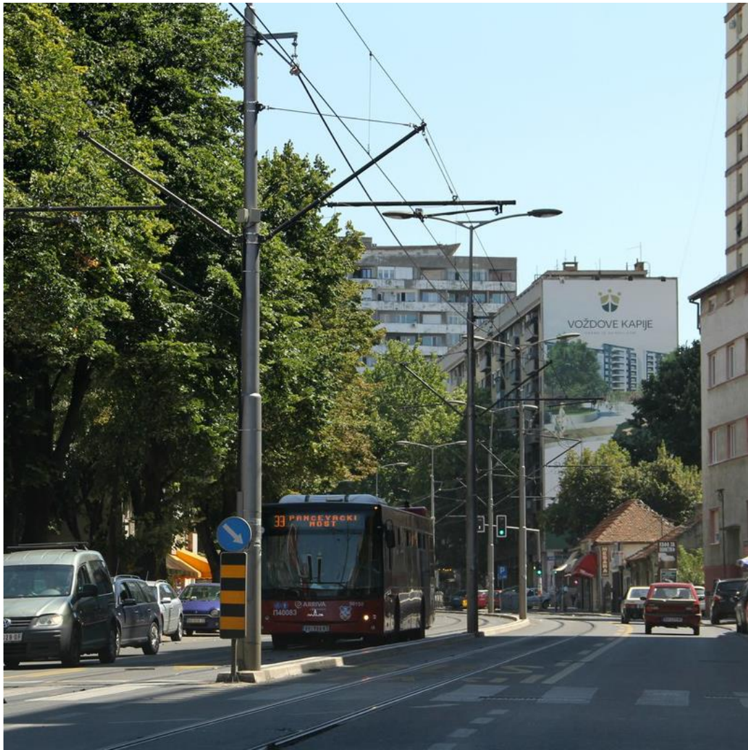
Figure 2 – Light Control System installed in Belgrade
