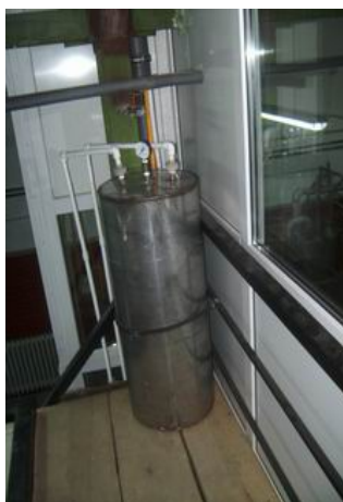
Figure 8 : Storage cylinder for biogas
