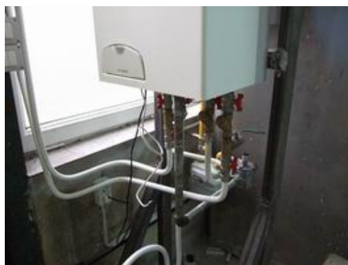
Figure 6 : The boiler used to circulate hot water trough the installation
