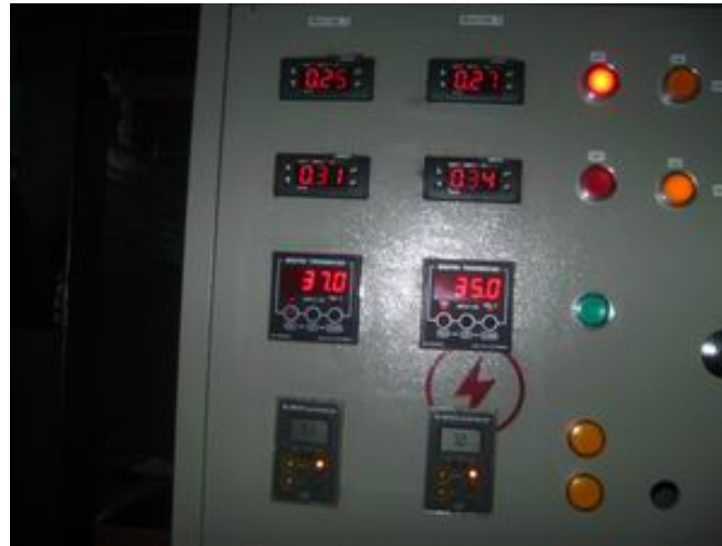
Figure 9 : Electric panel of the installation
