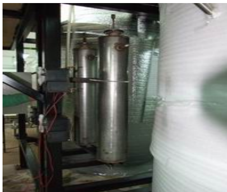
Figure 7 : The H_2S filter (in the back) and the CO_2 filter(in the front plan) of the installation, and also the dosing pump used for “washing”the CO_2 filter
